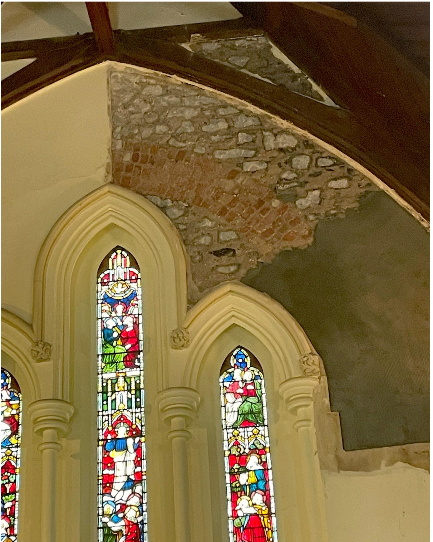
Ahead of today's 'update' on the restoration works in the church, please note this photo of the South Transept wall.
